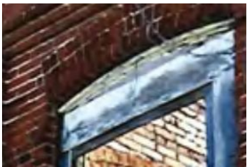
Window Frame Glazing putty
